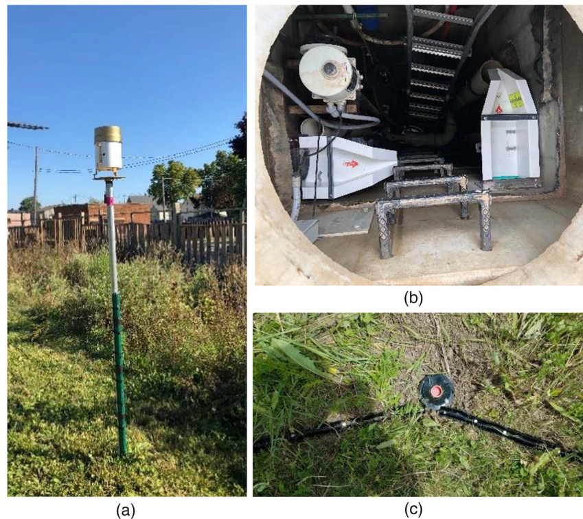
Fig. 2. (a) Tipping bucket rain gauge at Cream City Farms, with the north bioswale in the background; (b) view into manhole to junction box where two flumes measure underdrain flow from both bioswales; and (c) picture of influent sampling structure (plastic ground covering to prevent erosion around bottle not pictured). (Images by Elizabeth Regier.)
